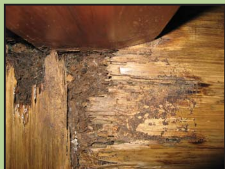
* Typical termite destruction
